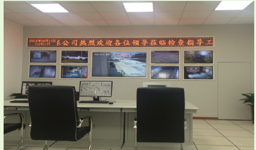
Centralized control room of the industrial solid waste disposal project
